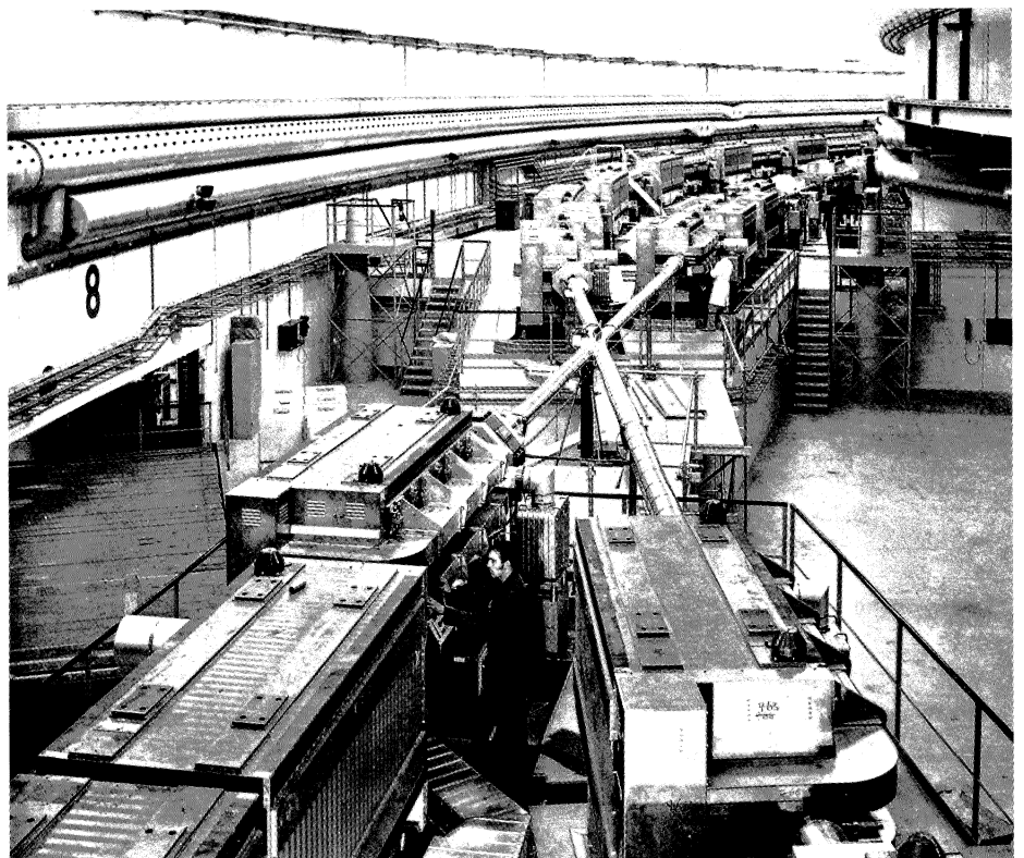
In the beginning. The bare ISR 18 intersection in 1970. Compare this with the photo on p. 96!
